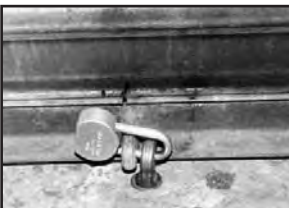
(Above) Bottom of gate is locked to a removable eyebolt in the sidewalk.
