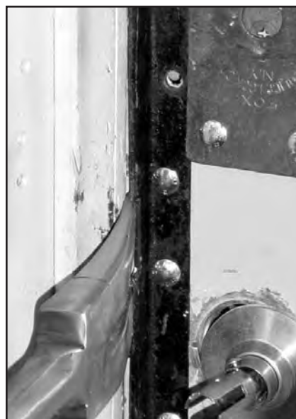
Figure #3--Drive the Halligan tool in until the tips hit the door.
