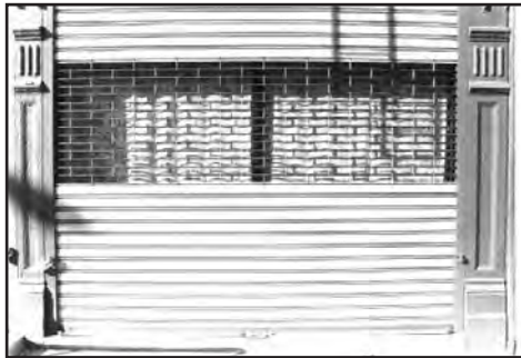
(Above) A combination gate with steel interlocking slats on the top and bottom and an open grill in the center. This gate is operated manually.
